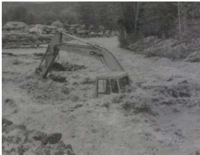
Figure 8. Excavator operator pushed into Coal Creek during the 1995 flood while building a temporary dike to protect Fernie's Airport subdivision. He was rescued from equipment. Credit: unknown.
