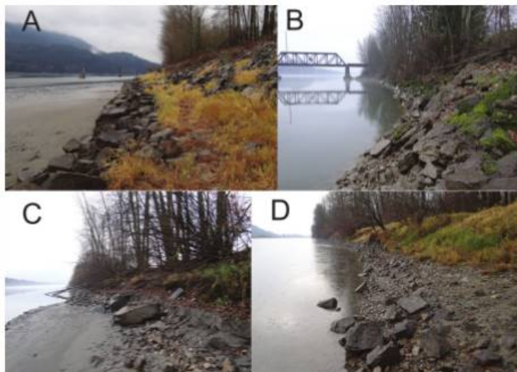
Figure 56. Examples of riprap application on lower Fraser River. Source: Reid and Church 2015
