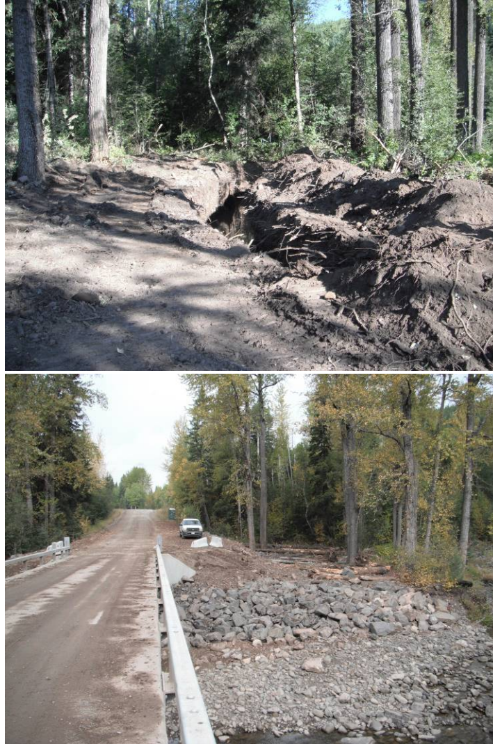
Figure 36. Setback rip rap trench to protect road from a channel migrating (to right of photo).
