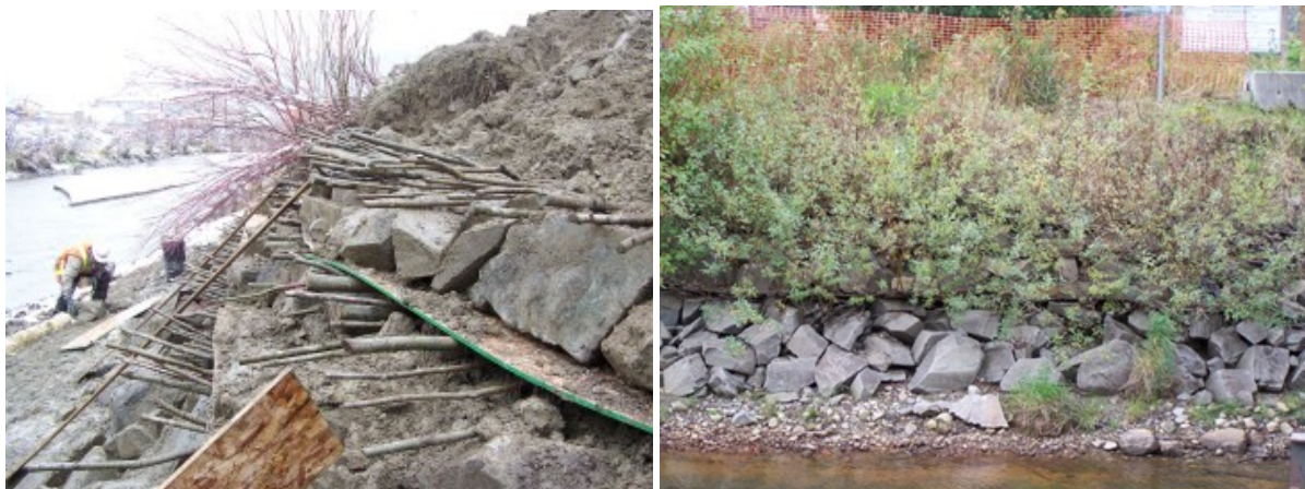
Figure 38. Vegetated rip rap installation – brush layer of live cuttings protected by plywood (left), vegetation growth two years after installation (right) (Photos: Terra Erosion Control Ltd.).
