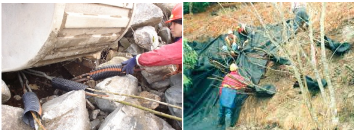
Figure 37. Examples of live cutting pockets being installed in rip rap (Photos: Terra Erosion Control Ltd.).
