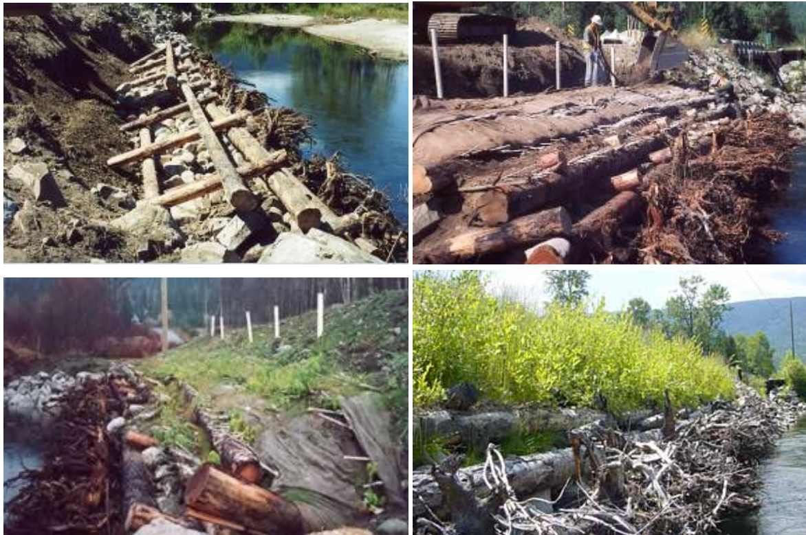
Figure 39. Log crib wall with vegetated lift to stabilize slope along the Inonoaklin River, Edgewater BC for Ministry of Transportation and Highways (Photos: Terra Erosion Control Ltd.).
