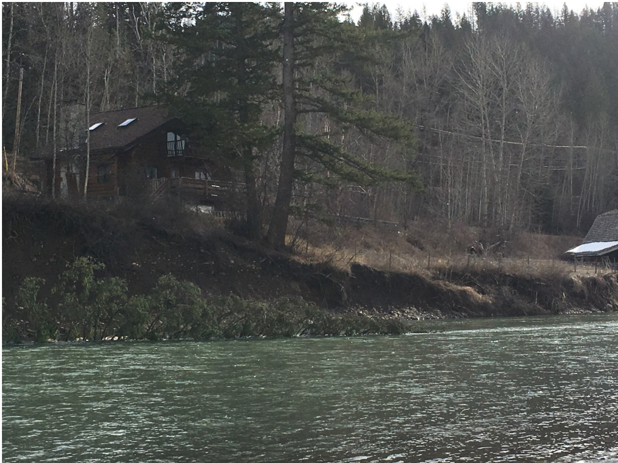
Figure 14. Downstream view of eroding bank (left downstream bank) and primary dwelling on property.
