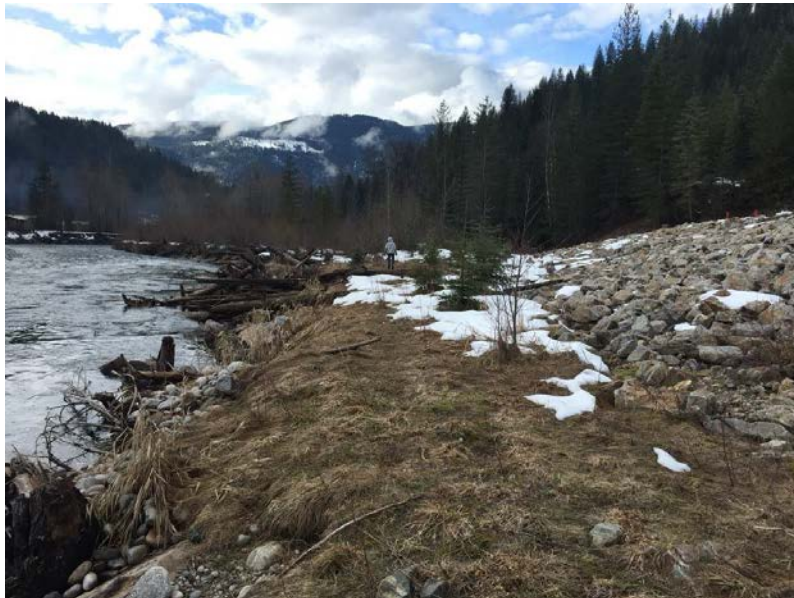
Figure 16. Example of tiered bank protection design with revegetated floodplain incorporated (Ymir, BC).
