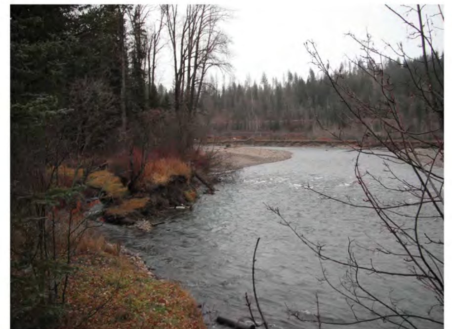
PHOTO 1: UPSTREAM VIEW OF BANK EROSION ON RIGHT DOWNSTREAM BANK (LEFT SIDE OF PHOTO).
