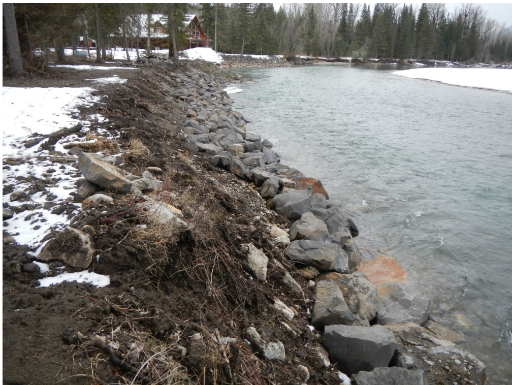
Figure 25. Rip-rapping along properties at the adjacent the Elk River along Thompson Road site.
