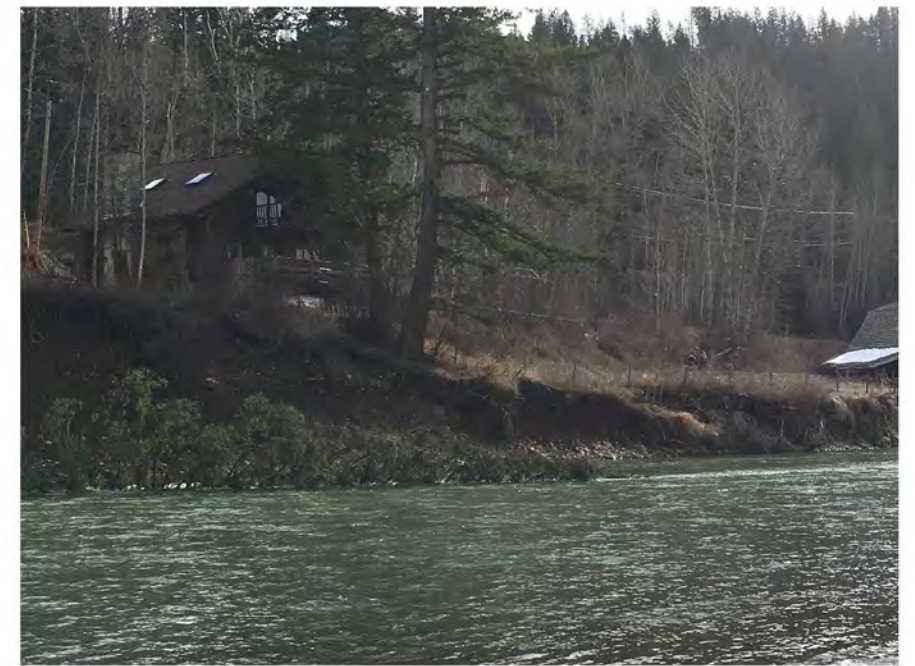
PHOTO 1: DOWNSTREAM VIEW OF ERODING BANK AND HOUSE ON SUBJECT PROPERTY.
